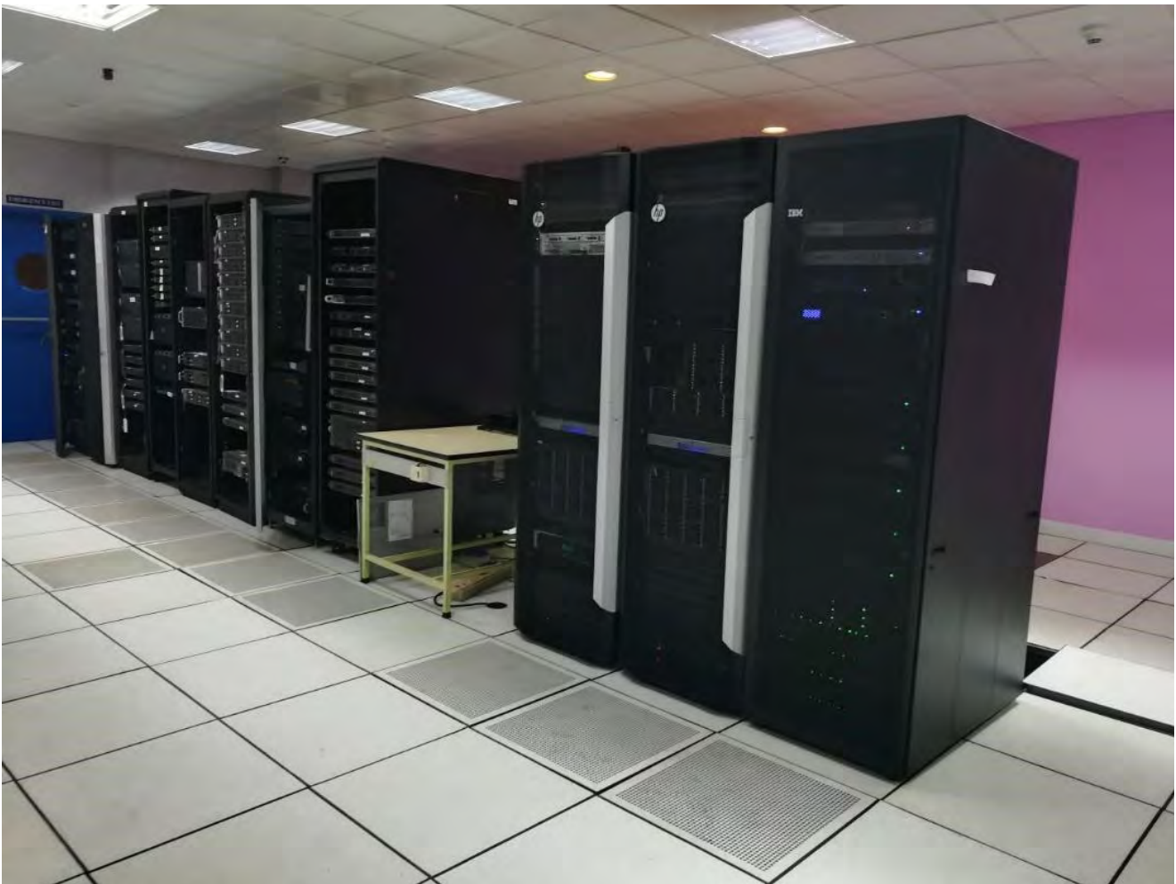
E-Services Server Area in the Data Centre
